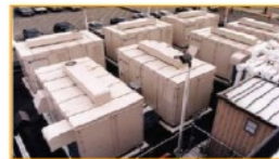
The 1.4 MW UTC fuel cell installation at Garden City, New York (picture courtesy of UTC)
